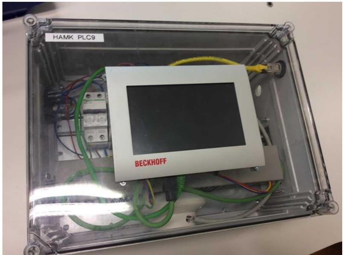
Figure 15. Beckhoff based PLC
