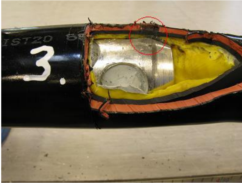
Figure 32. Example of failure at cone edge of connector (Laboratory report no.:1850S)
