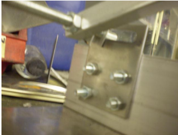
FIGURE 82 The fixing in place of the nut-bar is done with nuts on the nut-bar.
