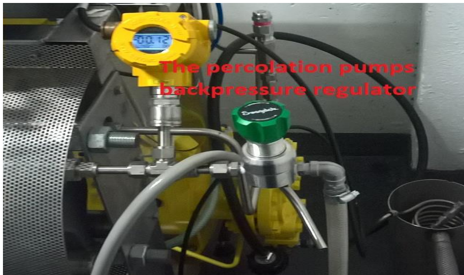
Picture 41. The percolation pumps draining backpressure regulator.
