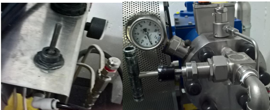
Picture 35. The membrane pumps activation switch.
