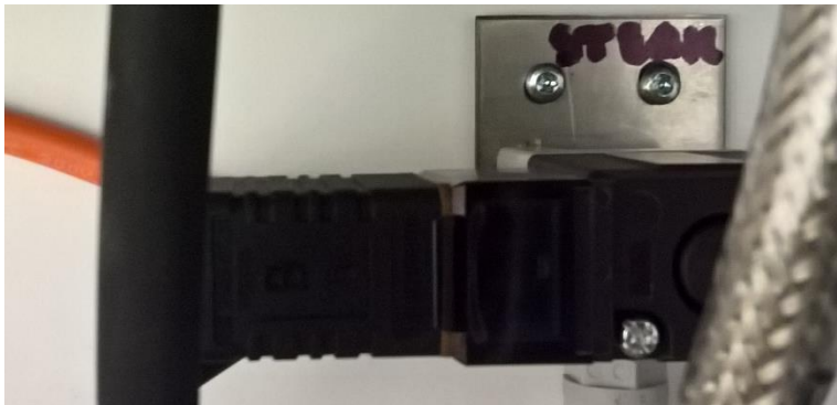
Picture 13. The pneumatic switch for valve SG1.
