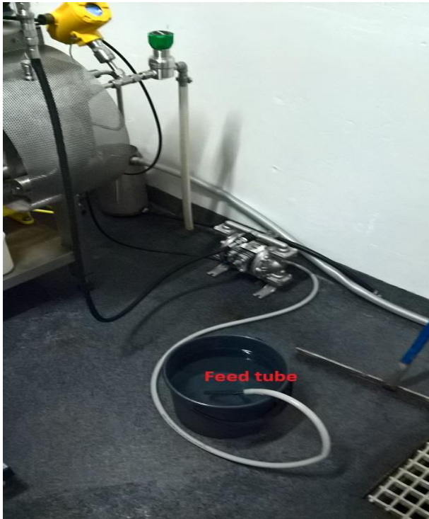
Picture 37. Example of a pumping process.
