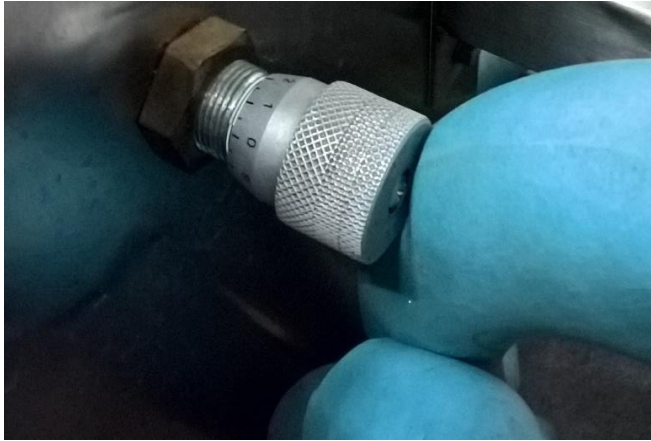
Picture 26. The hydraulic valve, placed on the right side of the reactors frame.
