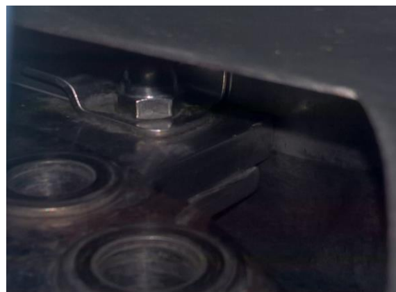
Picture 21. The containment cases bolts, which prevent dislocation.
