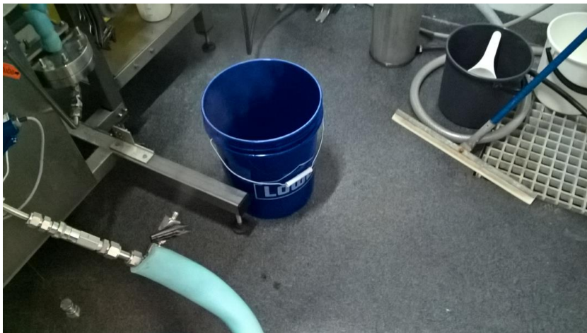
Picture 31. Steam being drained from valve SG3.
