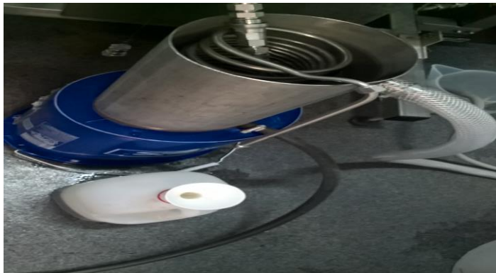
Picture 33. The reactors drainage line, linked to the quick connector.
