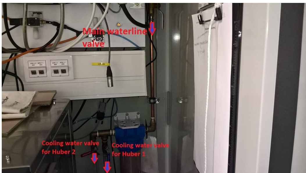
Picture 12. The Huber heaters waterlines and valves.
