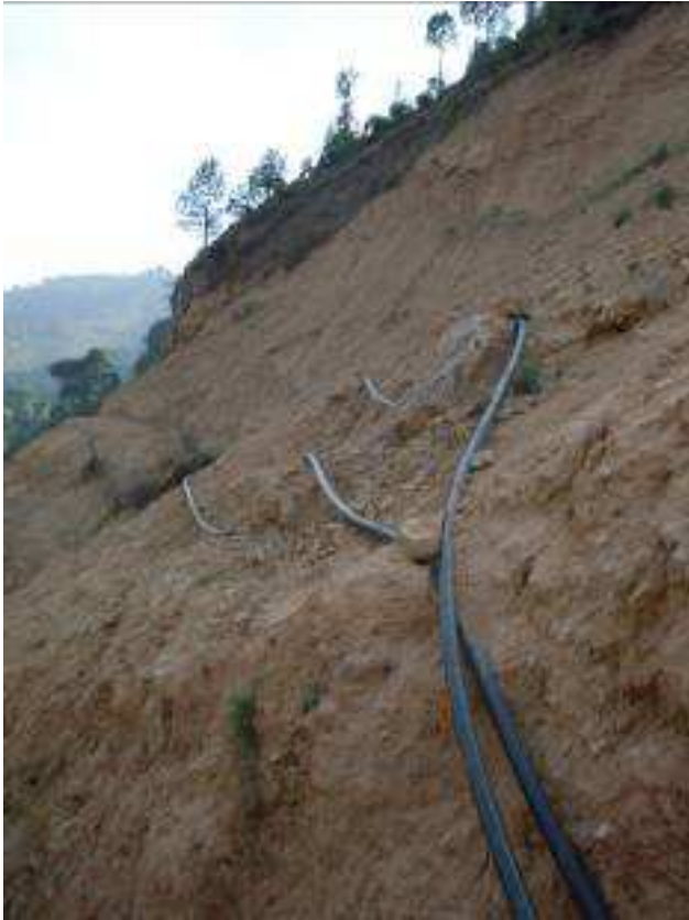
PICTURE 12 Water distribution pipes in Devichour [32]
