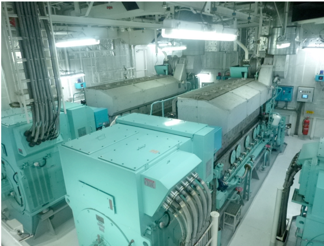
Picture 2. This pictures shows the auxiliary engines. (photo Jonas olin)
