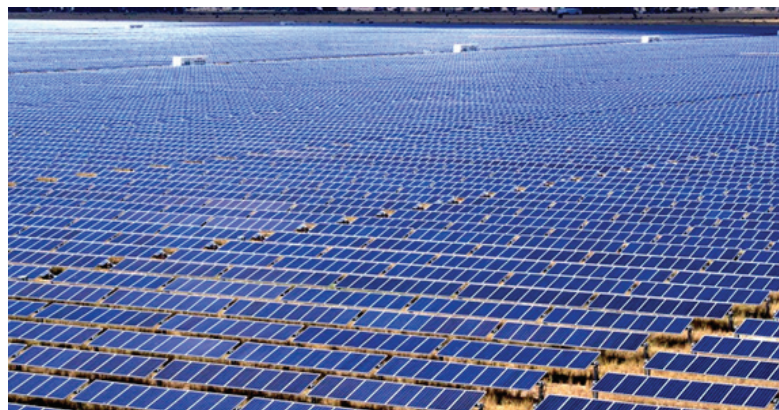
Figure 15: The Benban solar park (Mbogo, 2018)
