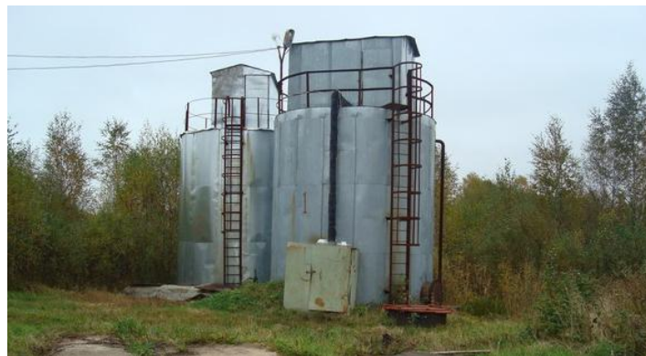
PICTURE 3. The technical conditions of raw water tanks on the site.
