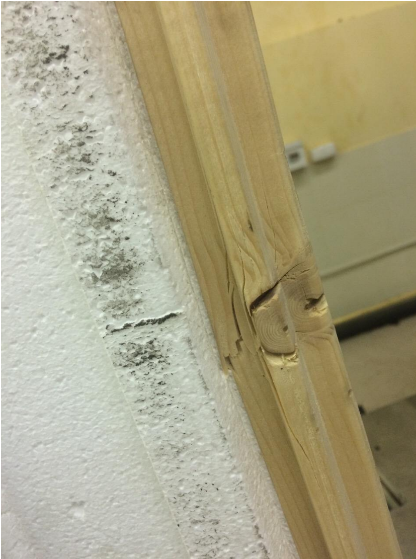
Figure 64. Destruction in the compressed zone of wood
