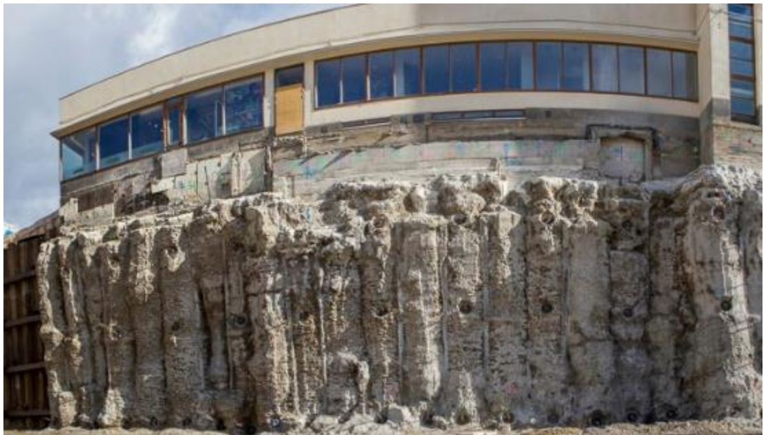
Figure 50. Retaining wall executed with jet grouting Soilcrete and anchored. (KFS Finland Oy, 2019)
