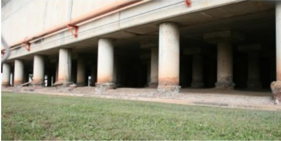
PICTURE 6. The corrosion caused by acid sulphate soil on a building (adapted from Queensland Government et al. 2013)
