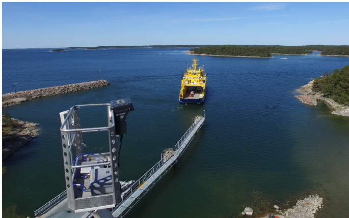
Fig. 3. The 700 MHz transmission antenna installed to a person lift at Kustavi shore.
