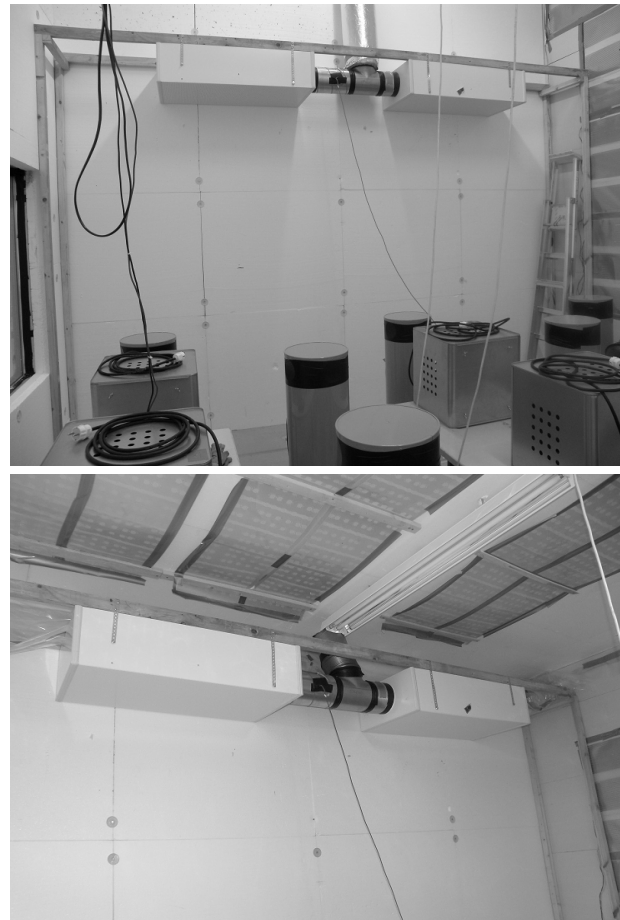
Fig. 3. Installation of displacement diffusers near ceiling in cases with 5.1 m (top) and 3.3 m ceiling height (bottom).
