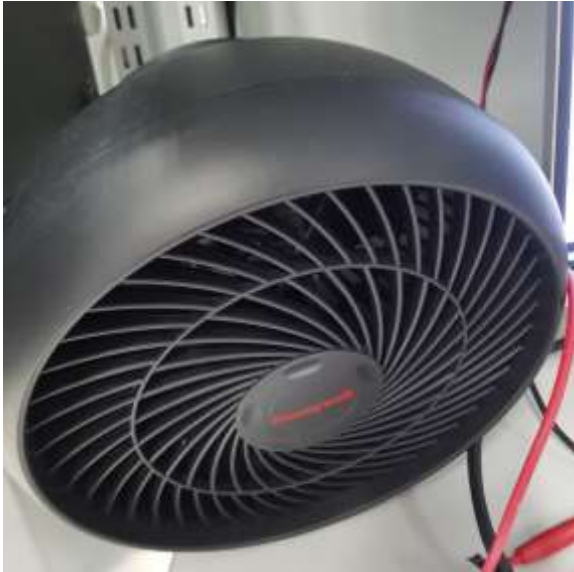
FIGURE 14. Currently used fan for cooling
