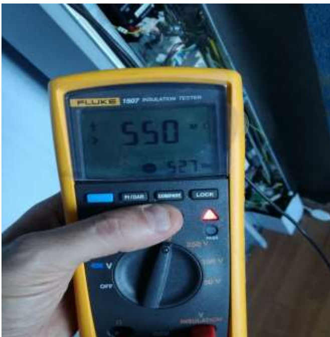
FIGURE 20: Insulation resistance measurement test results between PE and L terminals (15.)
