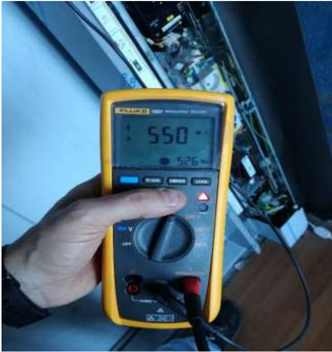
FIGURE 21: Insulation resistance measurement test results between PE and N terminals (15.)
