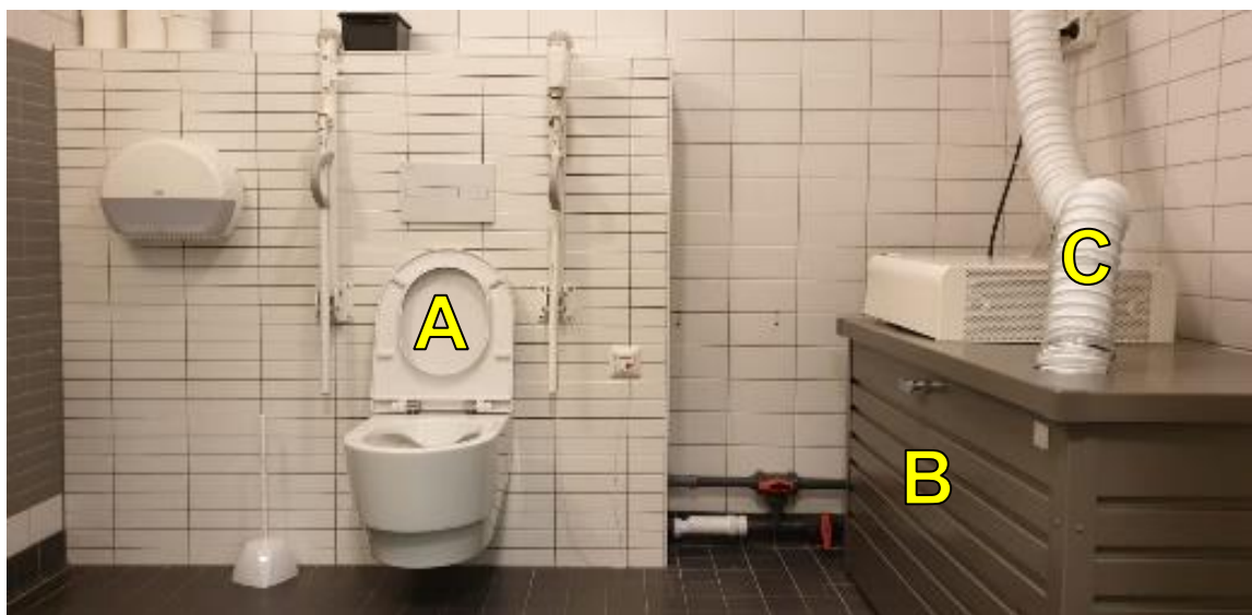
Figure 4. Alkaline urine dehydration setup at the Swedish University of Agricultural Sciences , with urine diverting toilet (A), dehydration container (B) and ventilation pipe (C)
