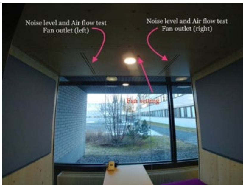
Figure 10 Measure air flow from the fan's air outlet and noise level caused by changing fan settings
