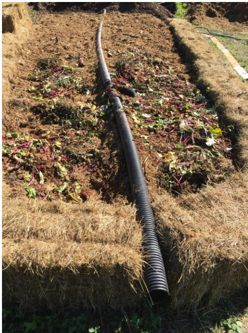
PICTURE 4. The aeration pipe laying on top of the first layer of feedstock. (Author 2020)
