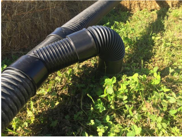
PICTURE 3. The aeration pipe connected with a T joint to the swage connection underground. (Author 2020)
