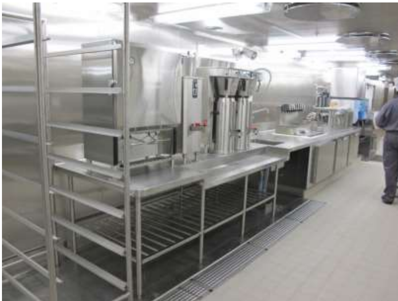
Picture 1. Tabletop equipment installed in previous project
