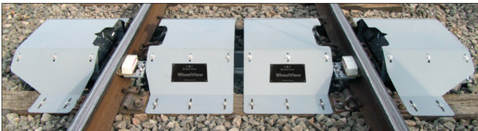
Figure 10. Wheel profile detector. (Trimble Inc, 2018)
