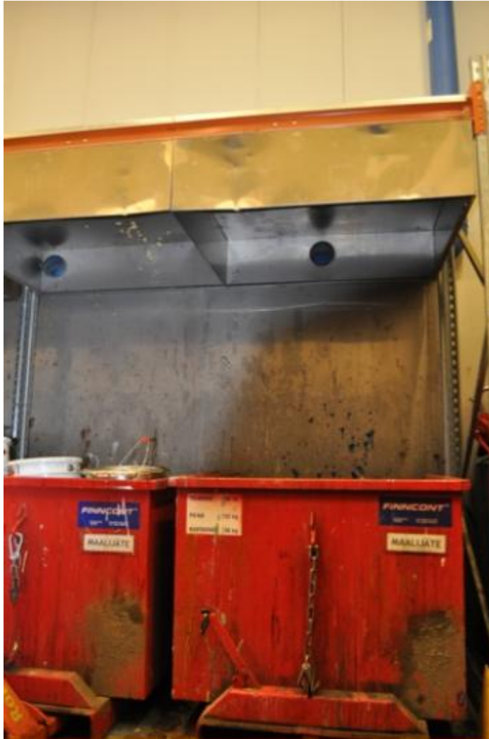
PICTURE 6: Ventilation system for paints
