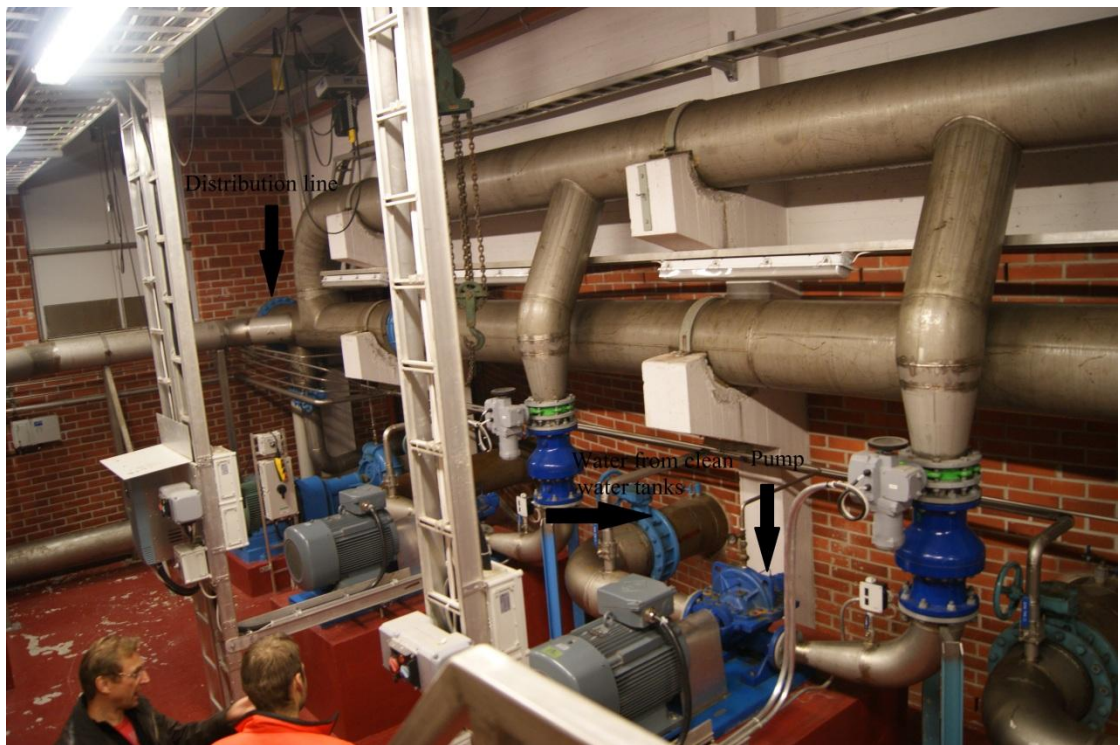
Figure 11. An engine room (a distribution line and a pump are shown)
