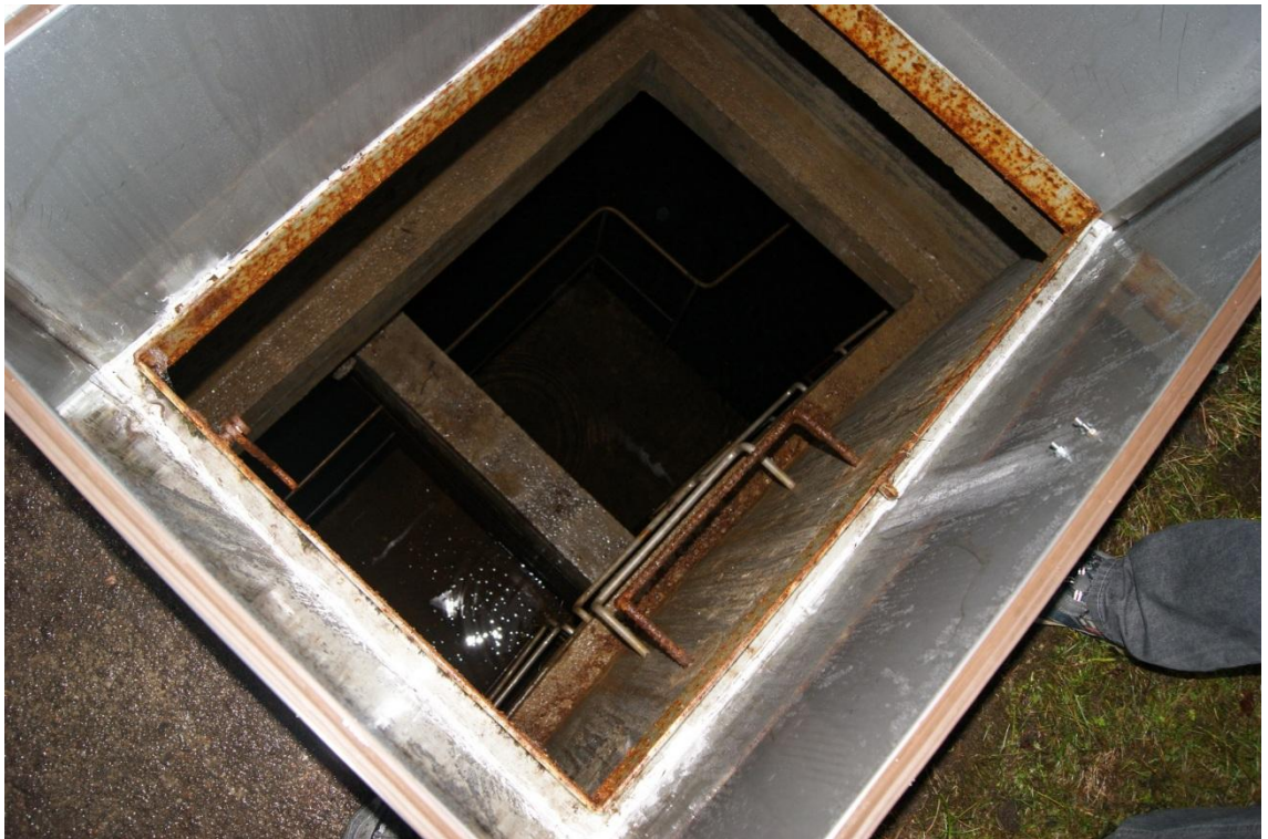
Figure 10. Manhole clean water tanks (situated underground)
