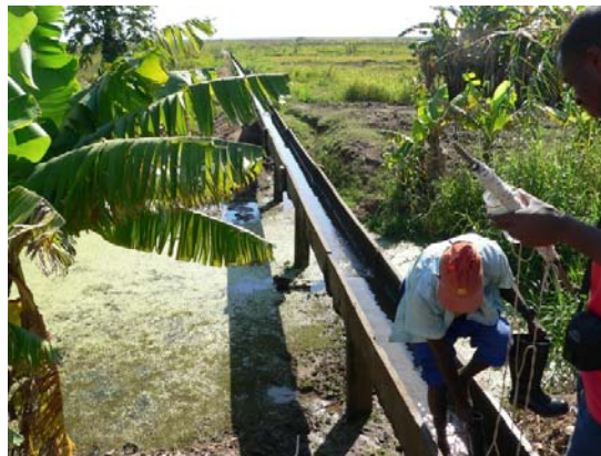
PICTURE 5. Part of the irrigation system in Chókwé (Source: Liisa Pekonen,2007)
