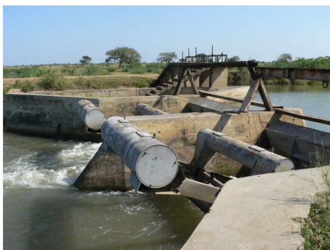
PICTURE 15. A small hydraulic structure in an irrigation channel to control water discharge (source: Liisa Pekonen, 2007)
