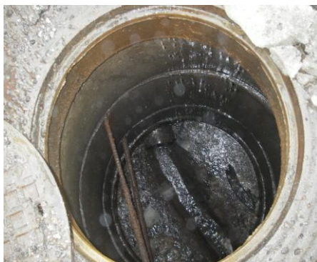
PICTURE 5.1 worn cast iron lid source inflow (Obijaju 2011)
