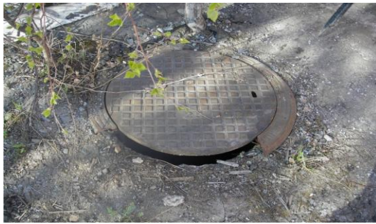
PICTURE 5.3 Broken cast iron frame source of Inflow (Obijaju,2011)
