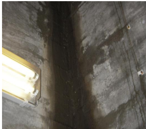
PICTURE 5.3 Infiltrations into a pump station (Peter Obijaju2011)
