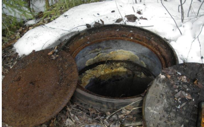
PICTURE 4.2 Concrete Manhole with a cast Iron (Peter Obijaju, 2011)
