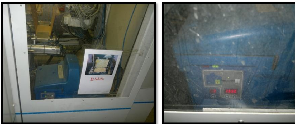
Figure 18 Views of the Glue heater situated in the WAM (Photo, Aduadjei 2011).
