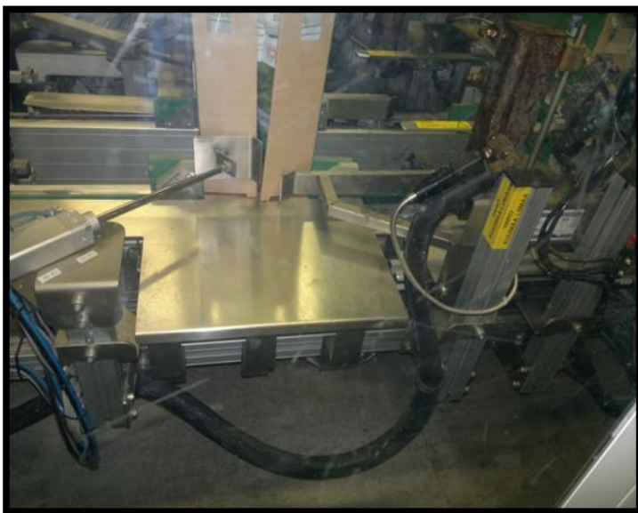
Figure 20 Glue pipe (black) running from the glue heater to the glue nozzle (Photo, Aduadjei 2011)
