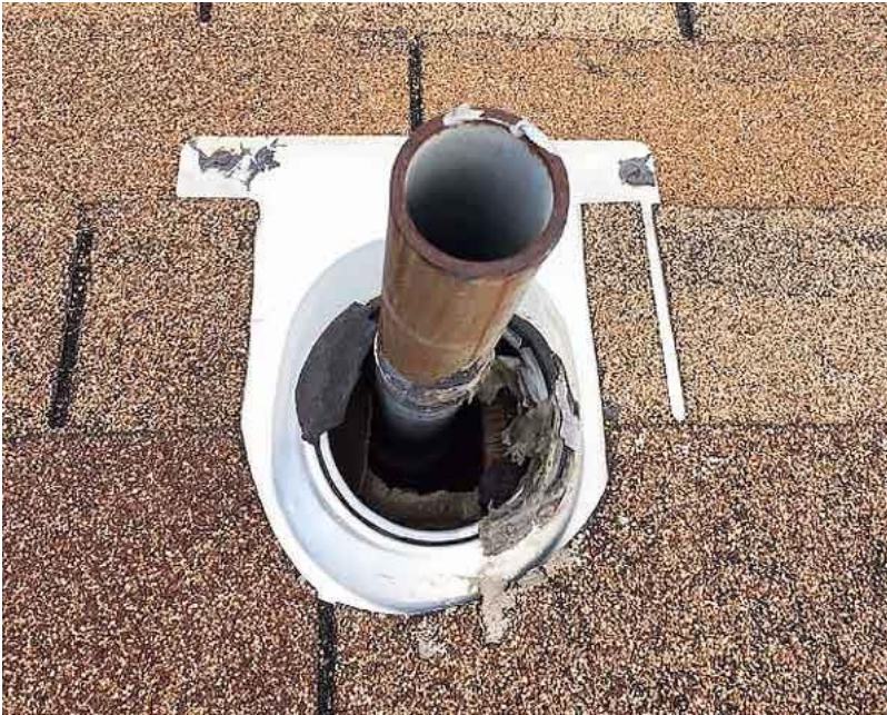
Figure 5. Roof duct moisture problem (918constructions 2020)
