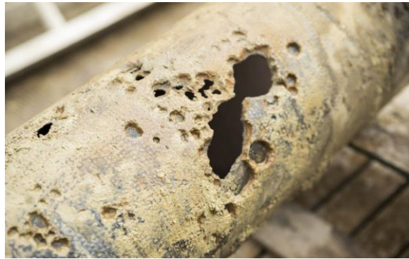
Picture 6: Pitting corrosion (Willey 2018)
