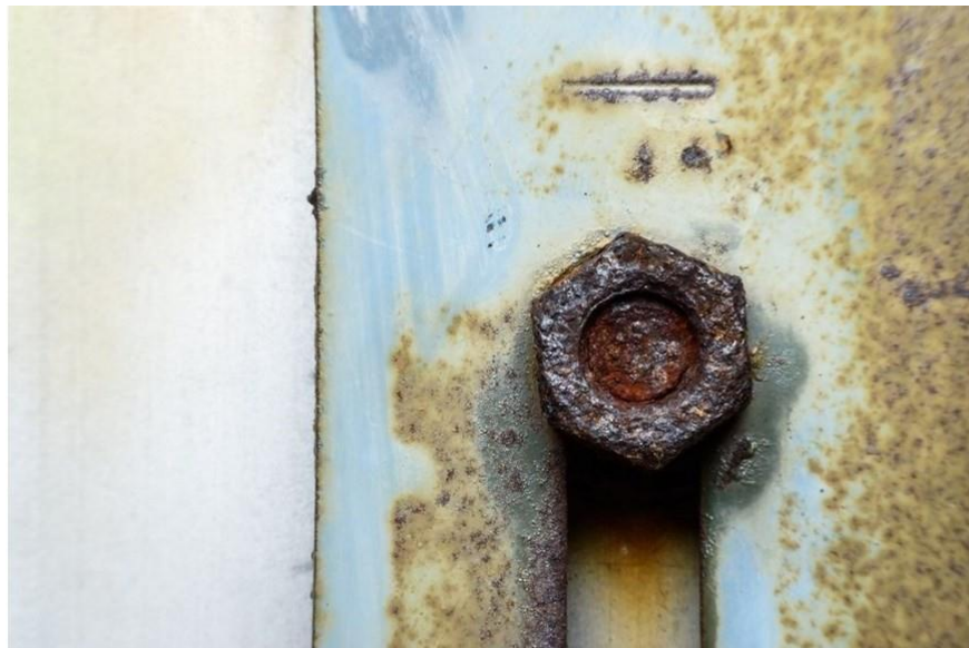
Picture 5: Crevice corrosion (Nanan 2018)
