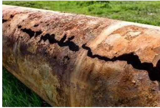
Picture 2: A corroded pipe (Dicoot 2017)
