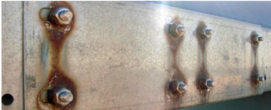
Picture 4: Galvanic corrosion (Belmont, 2018)
