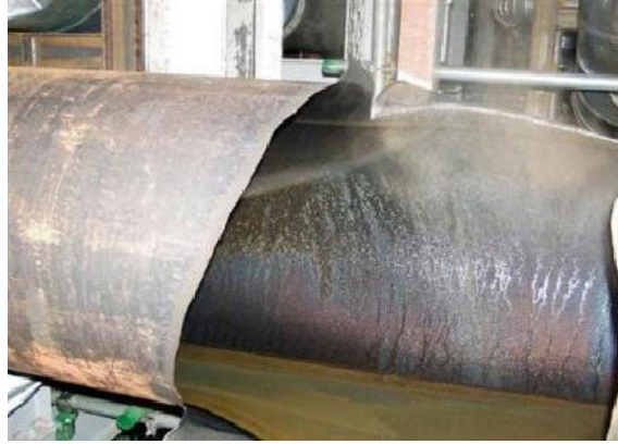
Picture 8: Transport pipe destroyed as a result of corrosion (Roberge 2007)
