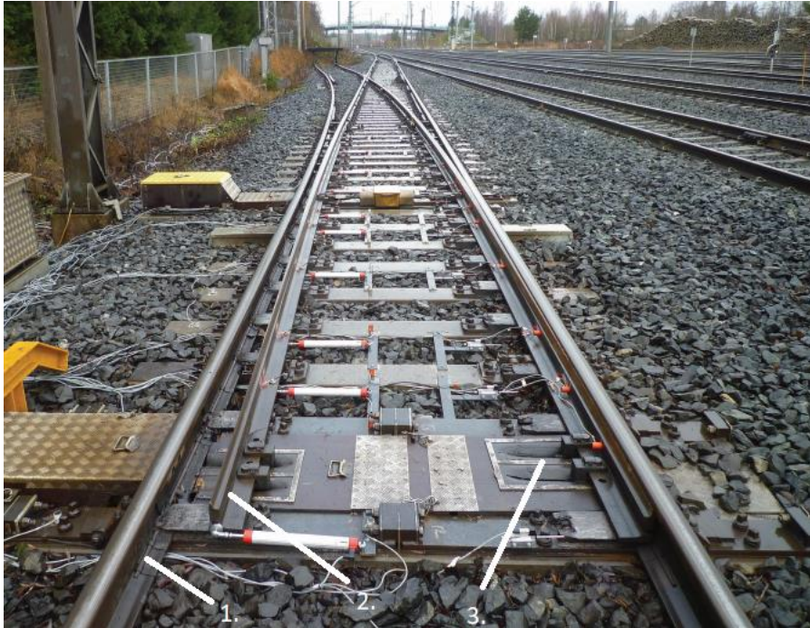
Figure 3. Switch heating resistors in a switch. 1. Support rail heating resistor 2. String heating resistor 3. Reversing rods pit heating resistor under the snow protector panel. [5.]
