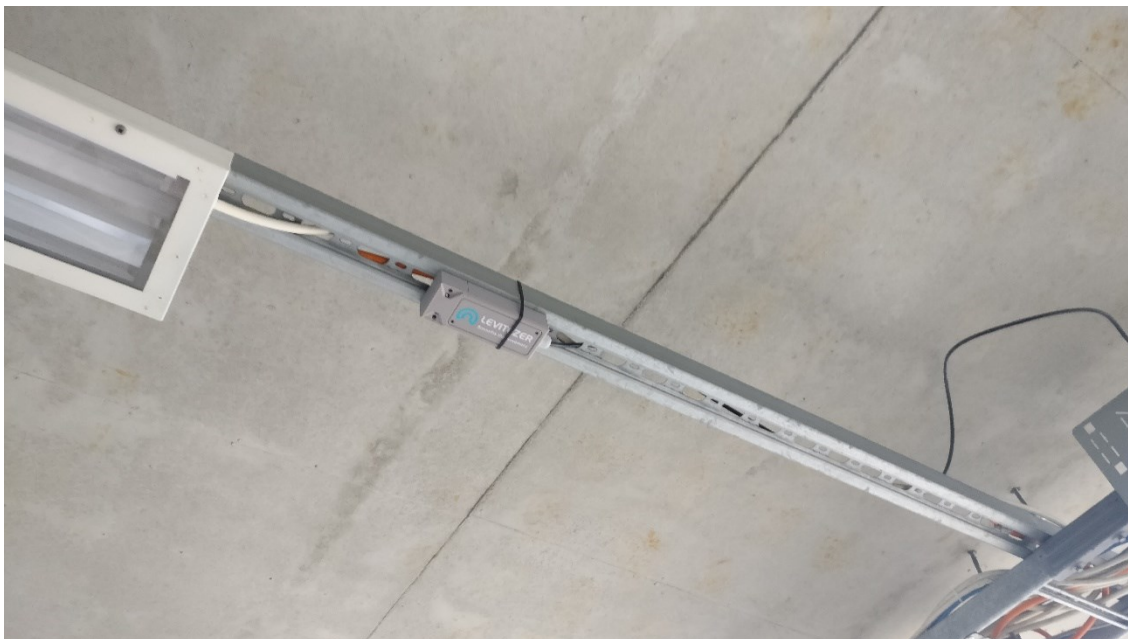
Figure 20. A close-up shot of the thermal camera device installed at the ceiling of the parking garage using zip ties.
