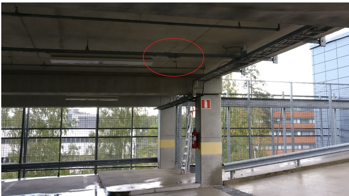
Figure 21. A Dual Thermal Device installed at the ceiling of the garage (see red circle).
