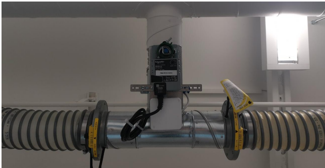
Figure 11. Connection of the air hoses to the main ventilation system
