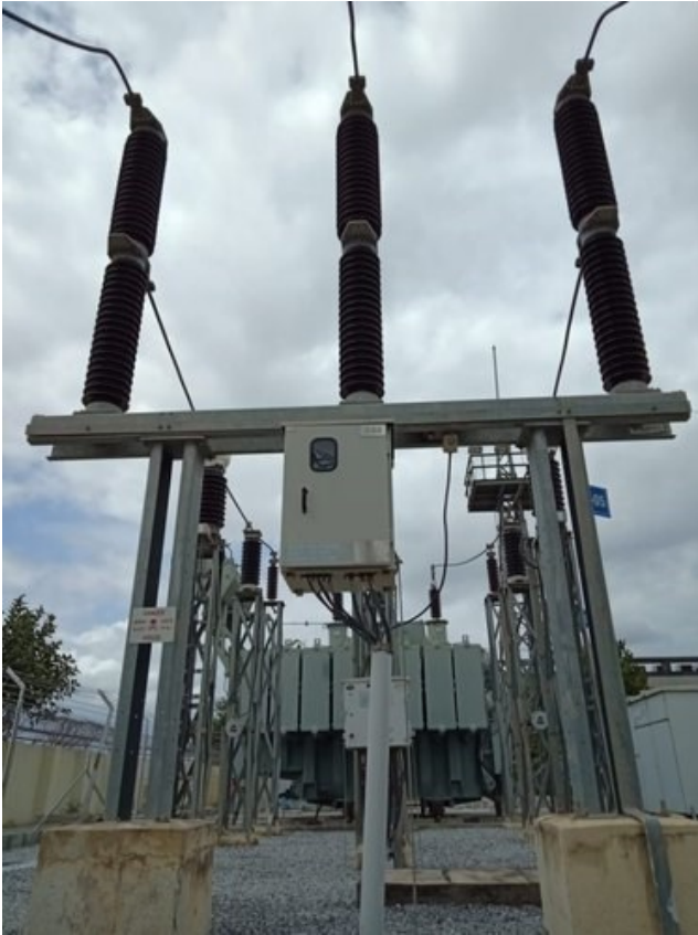
Figure 2 - Circuit breaker with SF6 gas chambers
