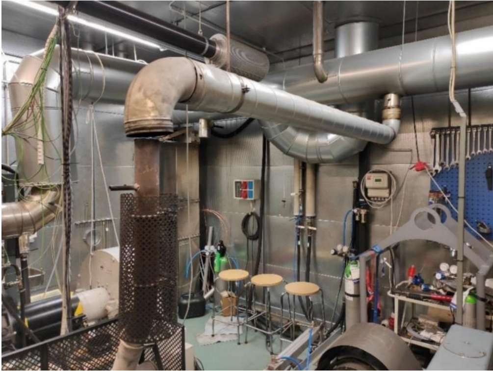
Figure 4. Exhaust pipe connected to the ventilation.
