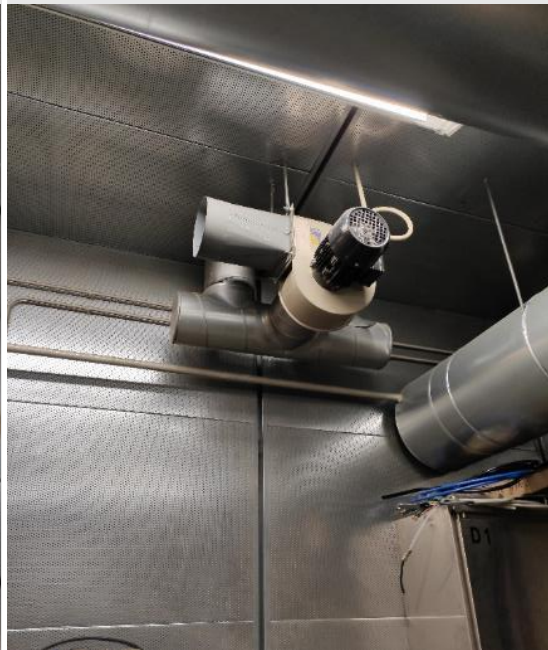
Figure 6. Turbine of the ventilation system.
