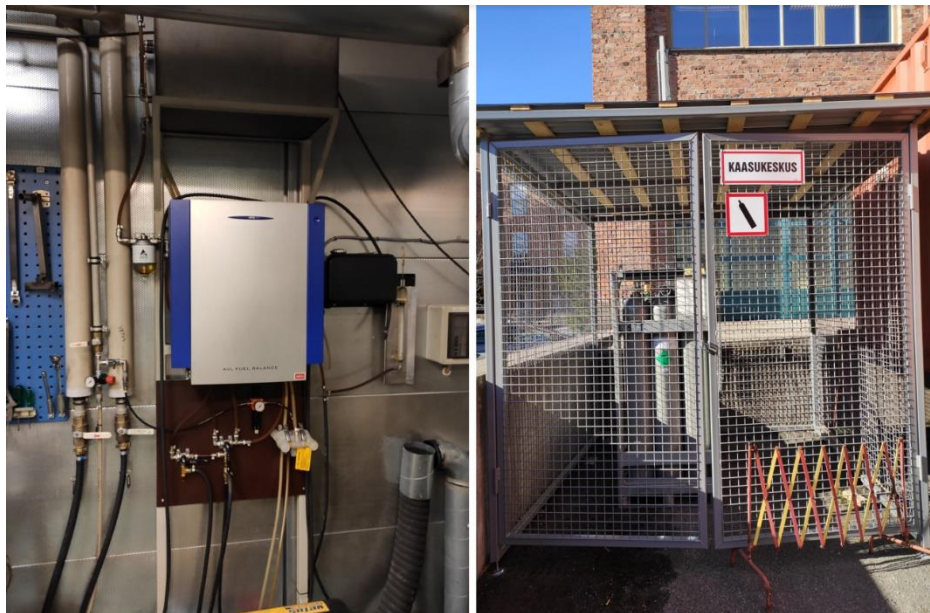
Figure 16. Current fuel tank installation and gas cylinders space outside in the engine laboratory in Novia UAS, respectively.
