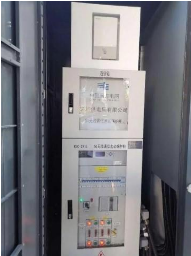
Figure 13: 5G wireless communication differential protection cabinet.
