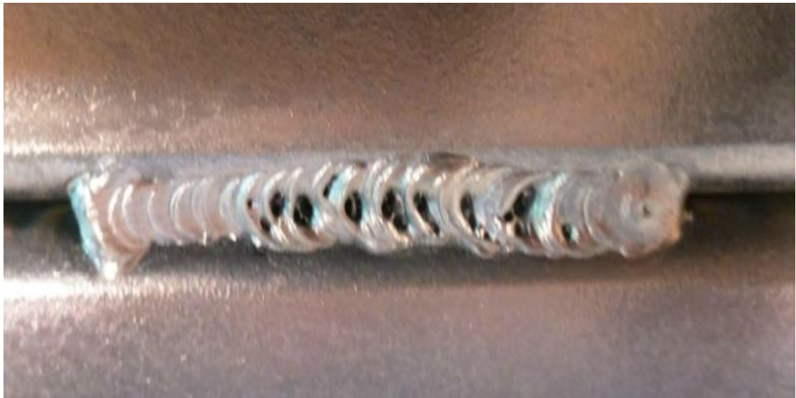
Figure 2 Bad Welding with holes inside
