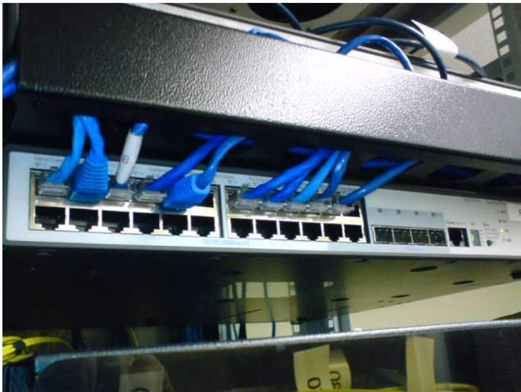
Figure 16. A rack mounted 24-port 3Com ethernet switch. (commons.wikimedia.com)
