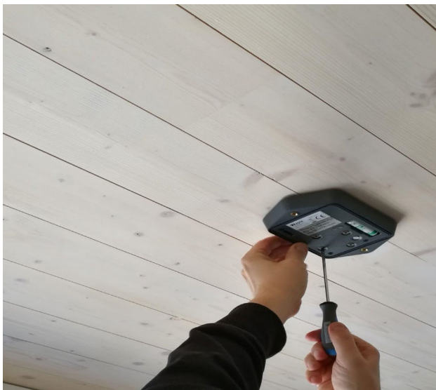
Picture 3. Fixing the sensor directly onto the CLT in the DAS Kelo building, Pirttinen Valterri LaplandUAS:
