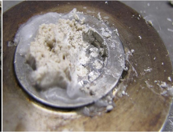
Figure 16. Clogged strainer plate. Photograph Christian Östman 2012.
