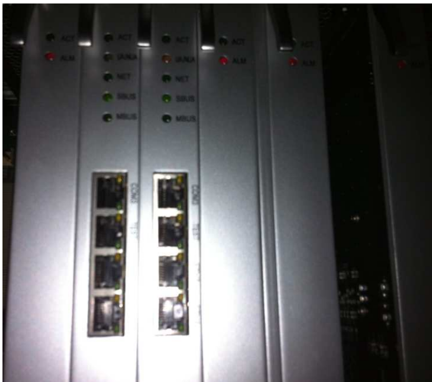
Figure 5.3. Near End SDH Equipment Panel.
