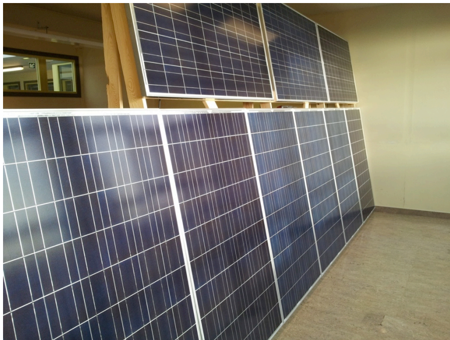
PICTURE 10. SE6M60 Monocrystalline panels installed in the classroom testbed
