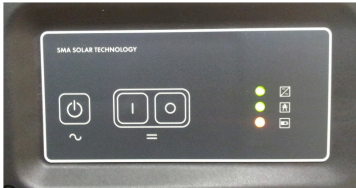
PICTURE 13. SI enclosure after startup with grid connected
