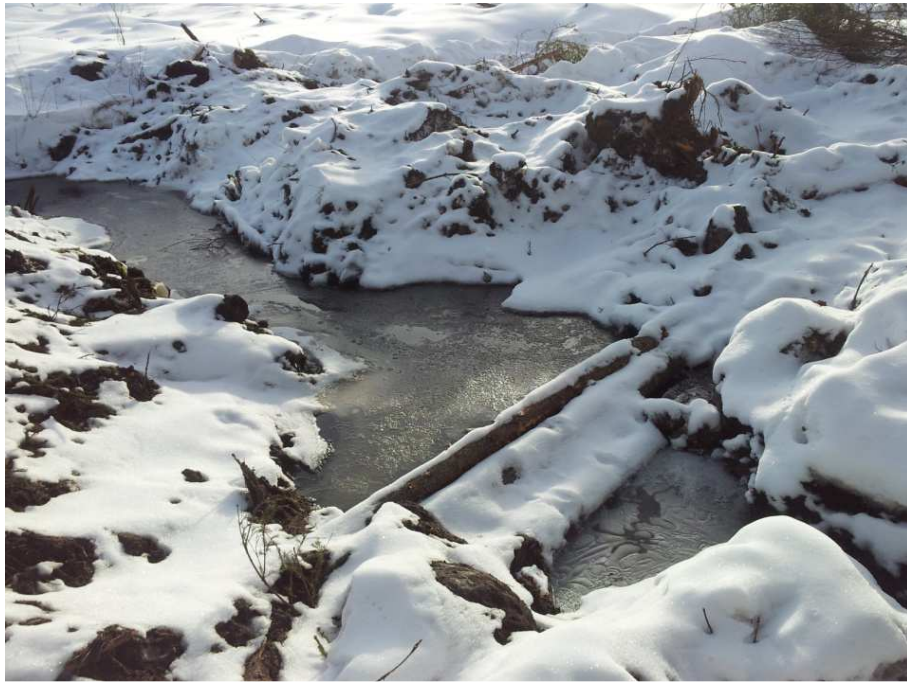
Figure 6 Submerged dam constructed in the point 4 of the plan. Water flows from left to right.
