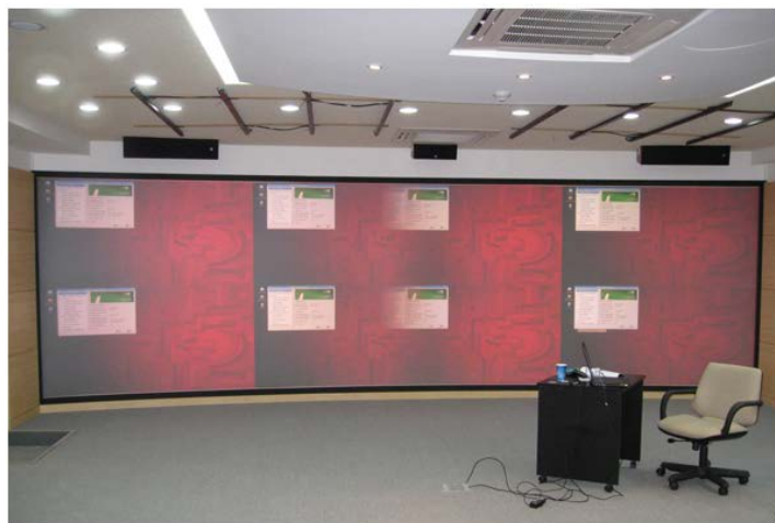
Figure 8. Example of front projected video wall system. /18/
