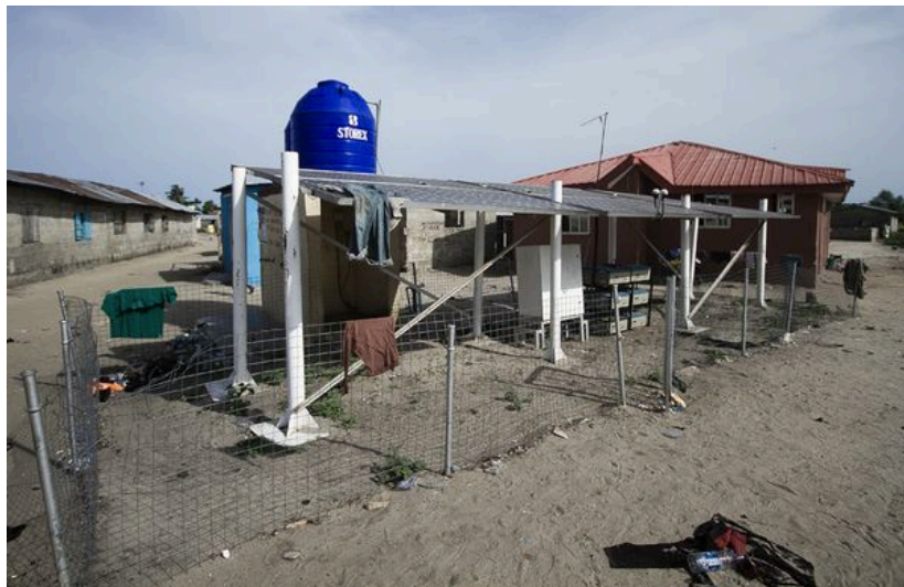
FIGURE 20: The Lagos state-sponsored solar powered Project at Onisowo village of Bishop kodji. (National geographic news)
