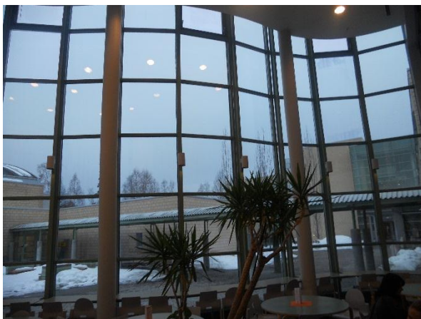
Picture 11. Area where the sun control window film was applied.
