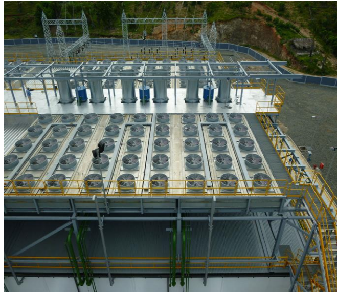
Figure 4. Radiator field and roof ventilation unit duct and damper.
