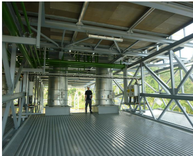
Figure 5. Roof ventilation units under the radiator field.
