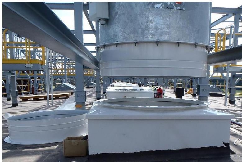
Figure 8. Example of a hanging fan. The galvanized steel part is the fan and under it is the removable joint.
