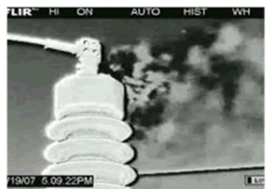
Elec. Circuit Brkr SF6 Leak
