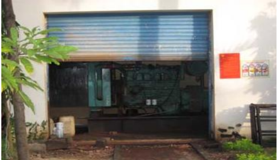
Figure 36 - Electric generator used at Thien Hai Son resort, Phu Quoc
