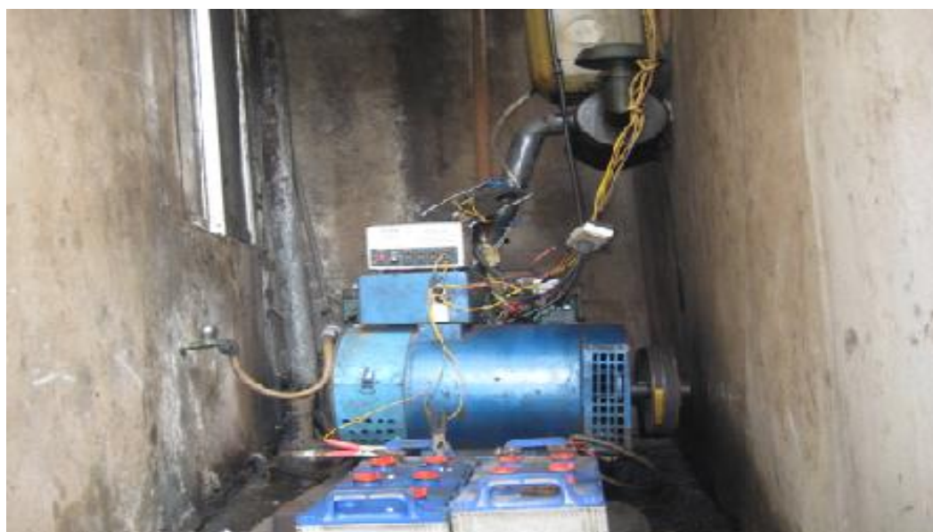
Figure 35 - Duc's electric generator in his house, Phu Quoc
