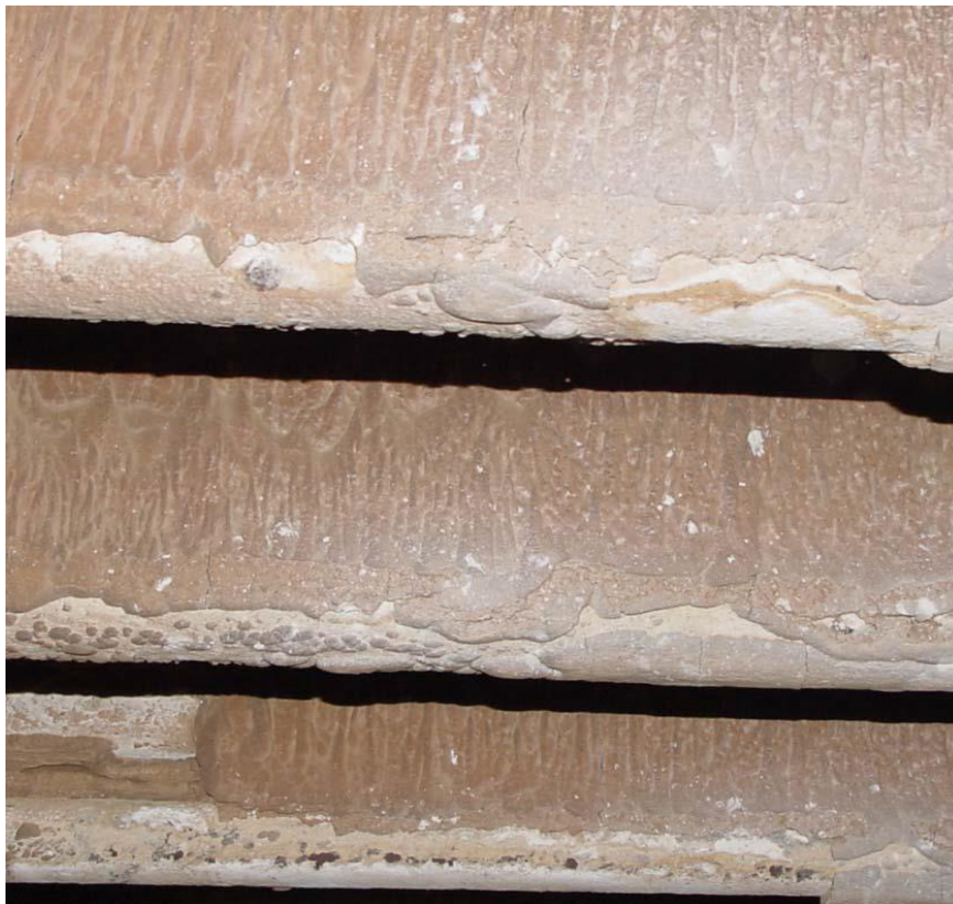
Picture 10. Fouled heat transfer tubes
