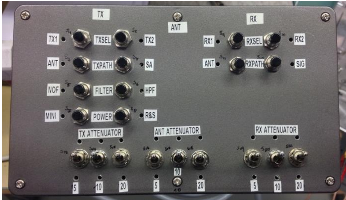
Figure G-2. Test Rack Remote Control
