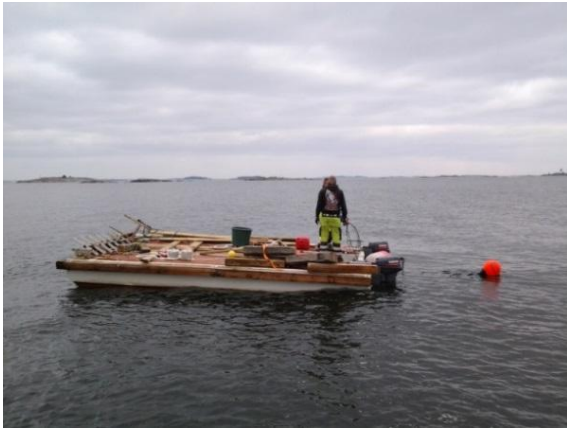
Picture 5: The mooring buoy of the Osborn & Elisabeth installed, June 2013 © Hanna Halonen
