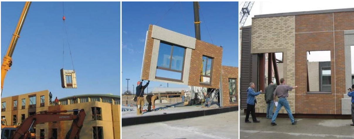
Fig 33: Construction progress on load-bearing wall section including glazing Source: McGraw Hill Construction (2011) – Combined by the author.
